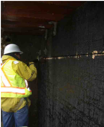
Figure 1-10: Span 1 girder 1 upstream face; end check at camp end.
