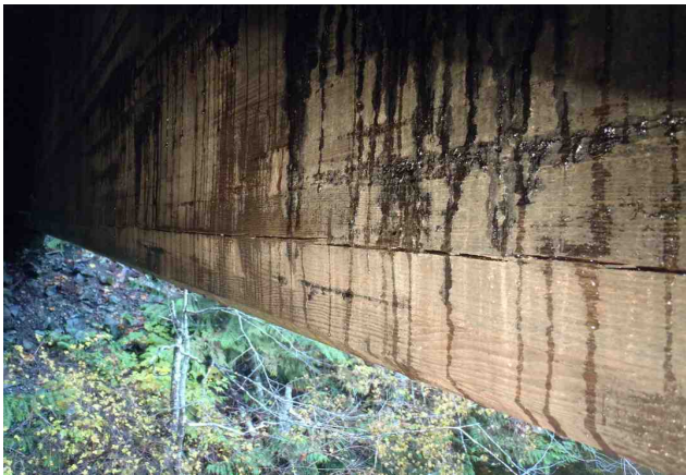
Figure 1-12: Span 1 girder 3 upstream face; check near bottom of girder.
