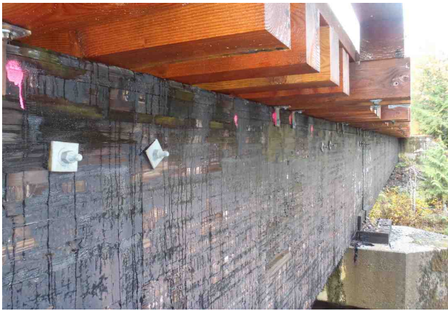
Figure 1-18: Span 2 girder 4 downstream face; longitudinal checks along the top of girder.
