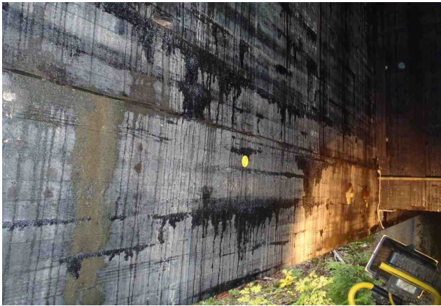
Figure 1-15: Span 2 girder 3 upstream face near mid-span. (AE2301-AE2302)
