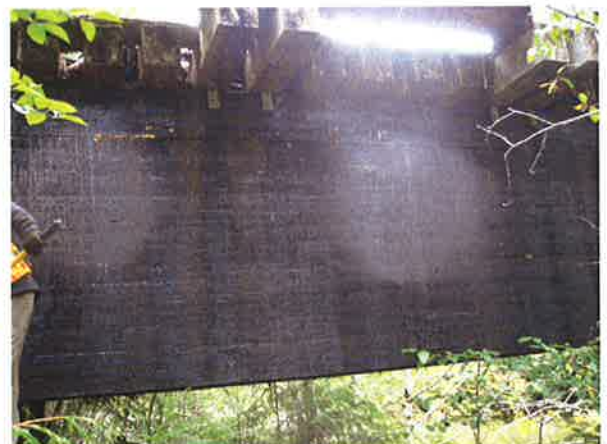
Photo 4 - Girder Crack near the Camp End Abutment
